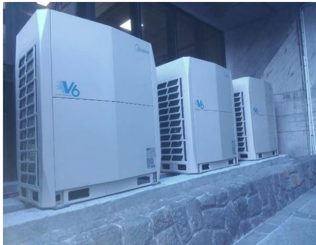
Energy-efficient Air Conditioning system
