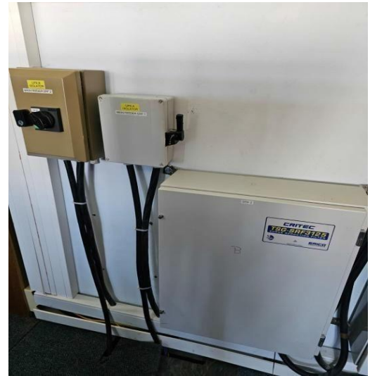
Fig 4: Output Panel for UPS
