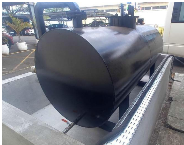
Fig 8: Bulk Fuel Tank
