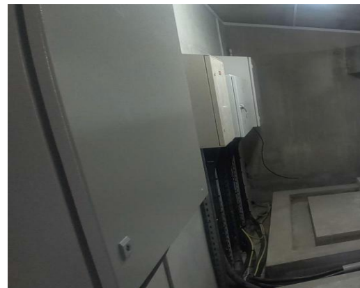
Fig 6: Changeover and Electrical Panels
