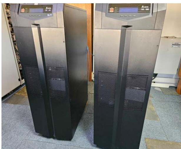
Fig 1: 30 kVA UPS at ACC Equipment Room
